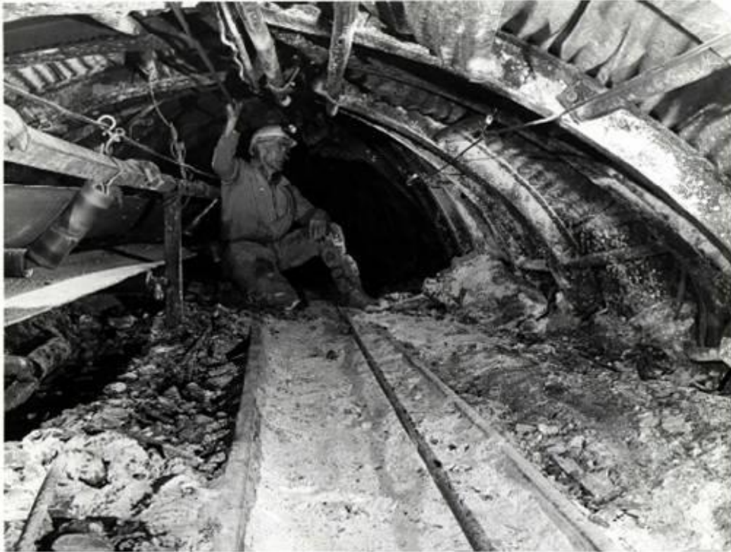
This photograph shows how the floor has lifted and has considerably reduced the height of the road. When this floor lift is removed it is called "beating up."
